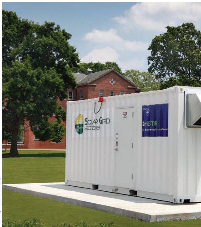
Courtesy: Solar Grid Storage
