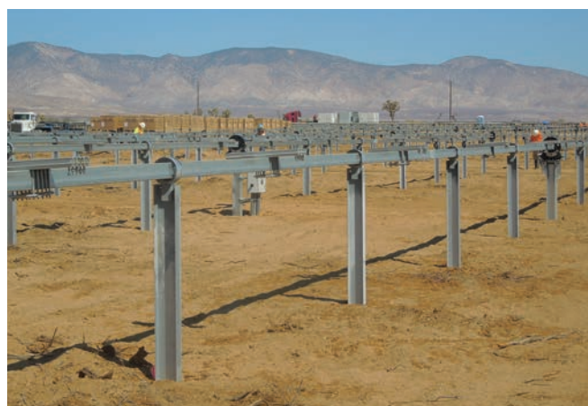
Courtesy Array Technologies
