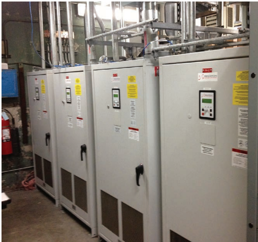
Courtesy Princeton Power Systems
