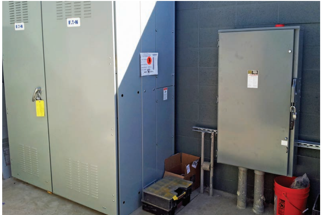
Location of OCP The new Section 705.31 requires that overcurrent protection for power-production source conductors, such as the fuses inside the disconnect on the right, be located within 10 feet of the point of interconnection, which in this case is at the switch gear on the left.
