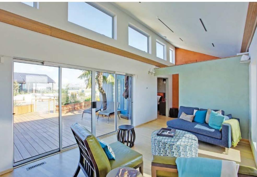
An in-ceiling hydronic system embedded in the plasterboard and barely visible in the home helps keep interior temperatures comfortable in the Santa Clara University team's home.
