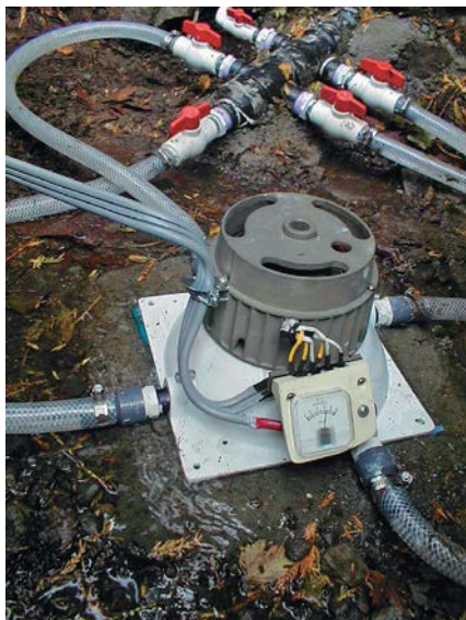
Upgrades like this one use manufactured components, while still keeping the budget low.
