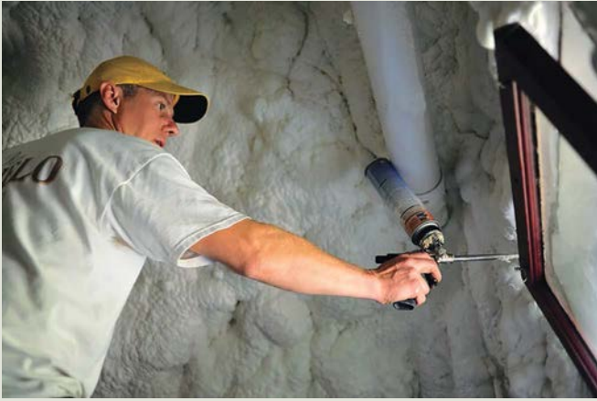
Added insulation boosts the home's thermal comfort and its overall energy performance.
