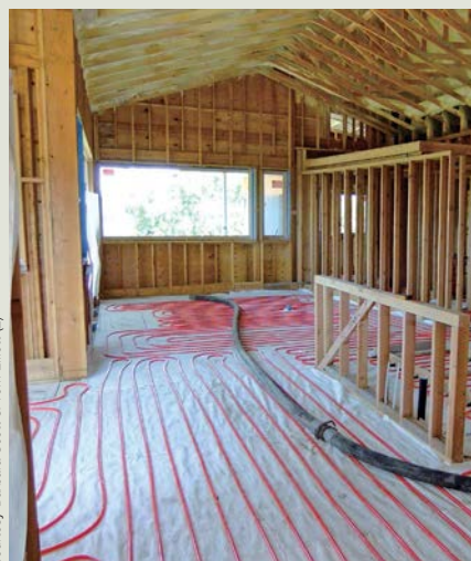
An eight-collector solar water heating system (not pictured) provides hot water for the hydronic floors.
