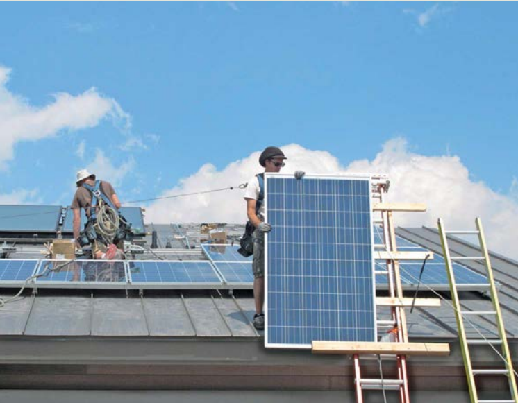
A batteryless grid-tied 14.8 kW PV system provides abundant electricity to meet the home and accessory dwelling unit's needs.
