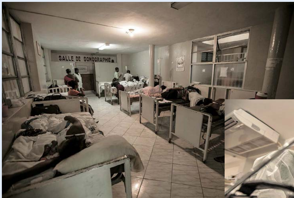
A battery backup system provides much-needed power for lights in a maternity ward (left) and for laboratory test equipment (below) in a Haitian hospital.
