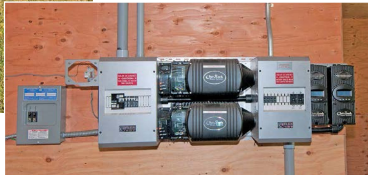
Below: The OutBack Power Systems dual VFX3648 inverters provide 7.2 kW of power for farm operations.
