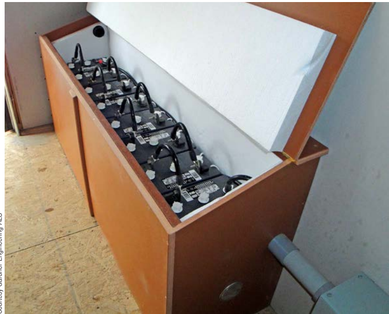
Courtesy Gardner Engineering ACS
