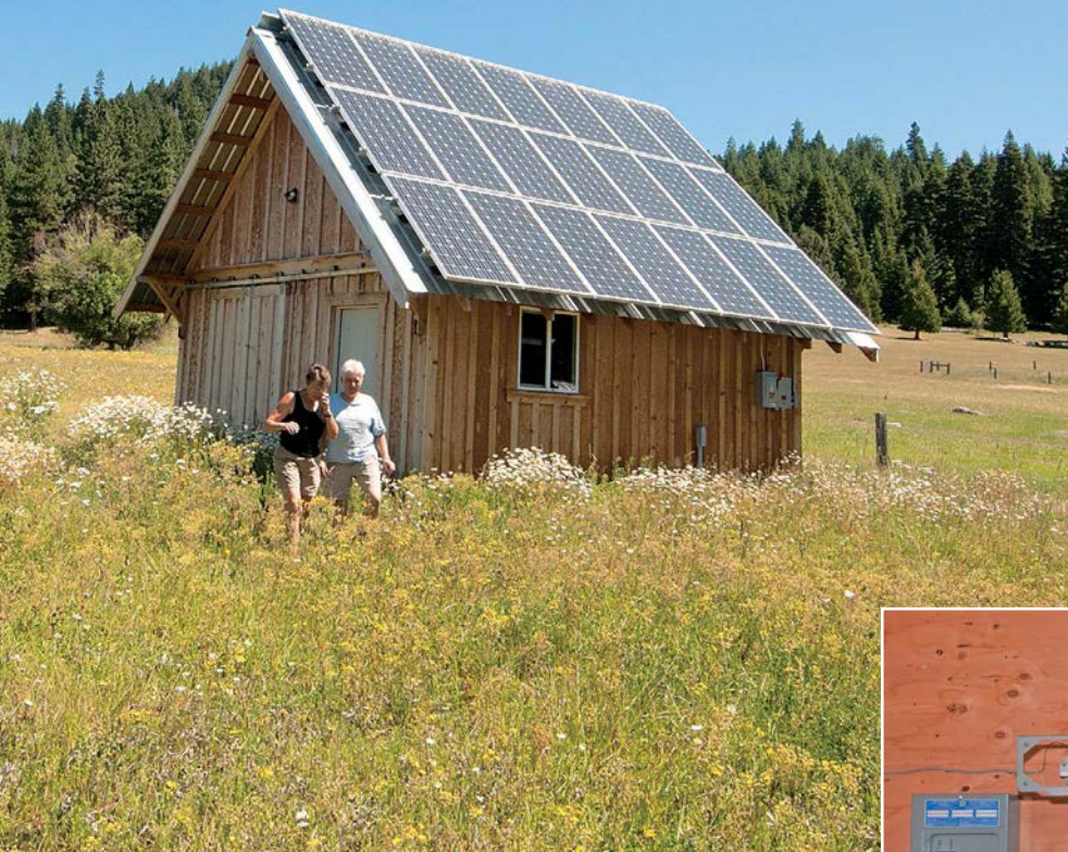
Left: The PV system on the barn has 21 Samsung 247 W PV modules for a total of 5,187 W. The system is mounted on a purpose-built power shed with a roof tilt equal to the site's latitude to optimize off-grid winter production.
