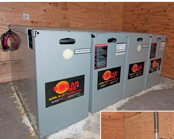
Left: Four HuP Solar-One 12 V industrial batteries, wired for 48 VDC, provide 1,690 amp-hours of storage capacity.
